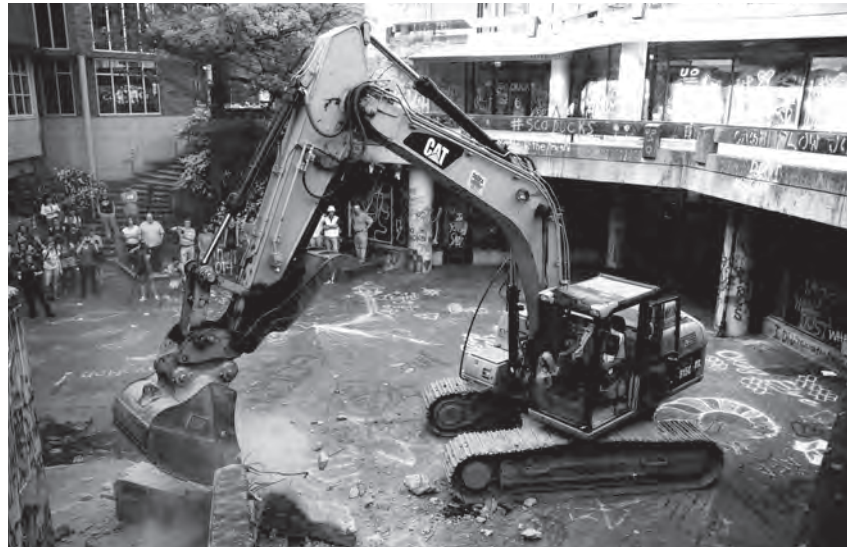
A Cat excavator demolishes a portion of the EMU courtyard steps to end the demolition event.
