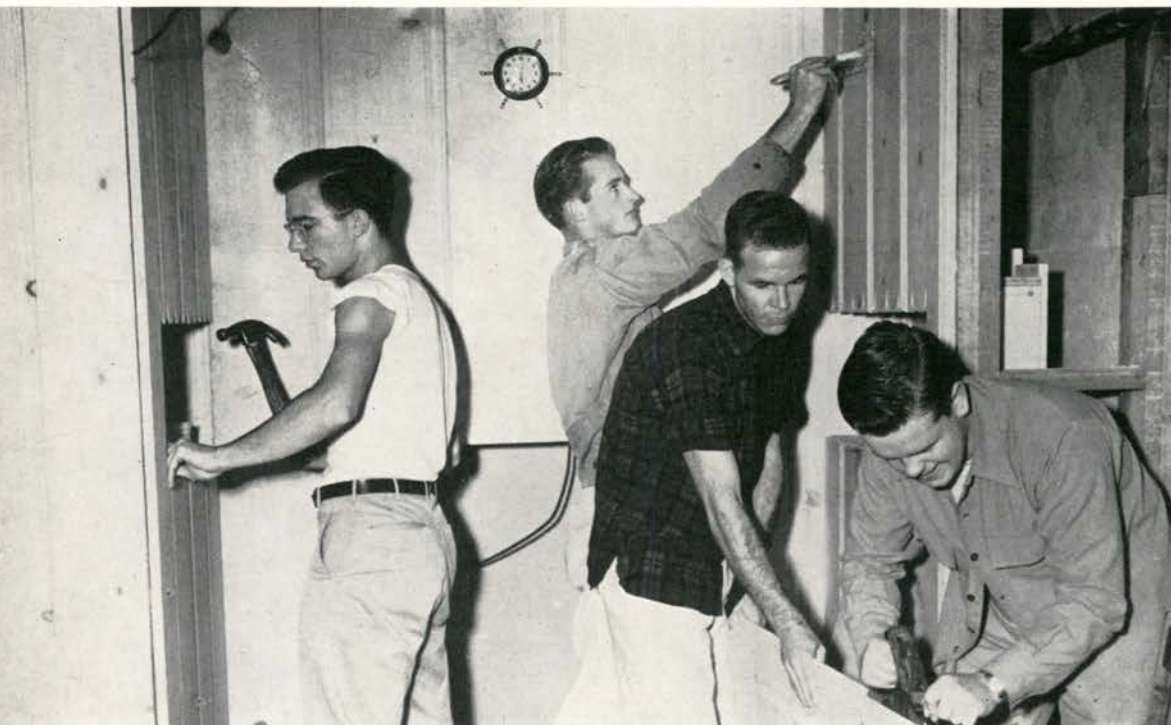
The DUs bring their carpentry ability to use, building their party room.
