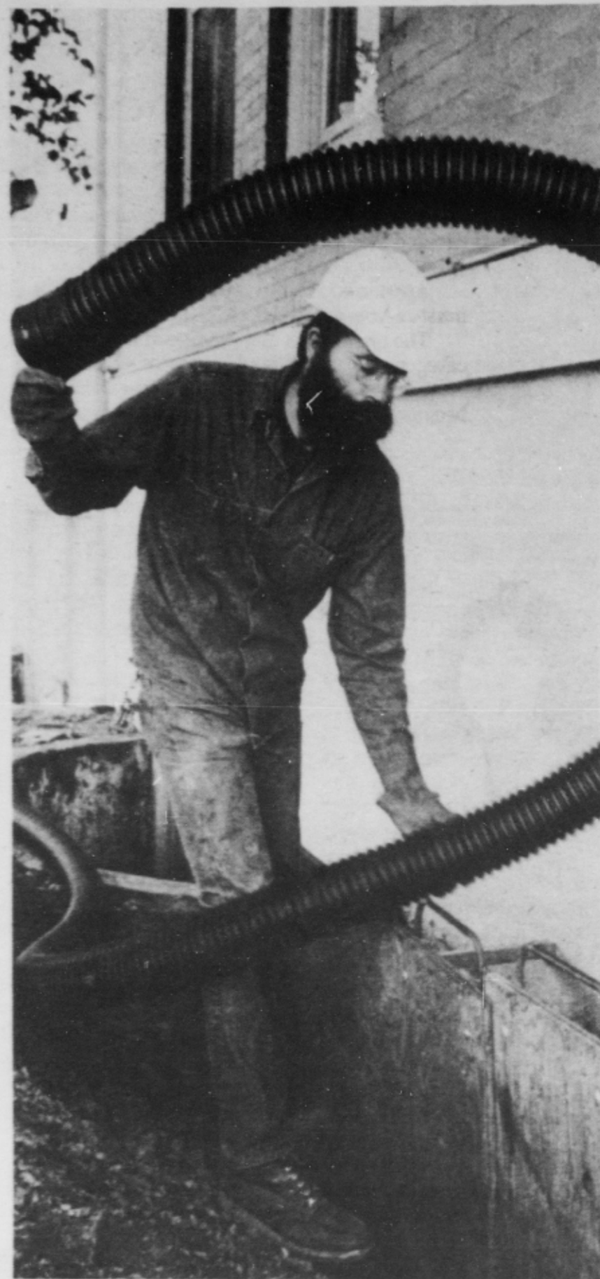
Rich Hill, Physical Plant employee, prepares to place a plastic drain pipe in the ground near Waldo Hall. The hall is plagued by basement flooding problems in winter months. The new pipe will correct the problem. (Photo by Tim Bernard)
