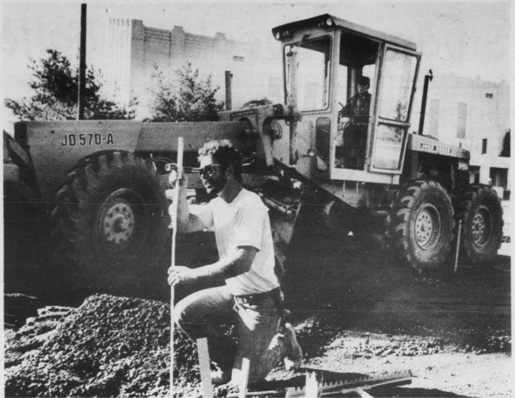
Mike Carroll, foreground, of Wildish Corvallis Construction Company, works on an extension to the Finley Hall parking lot. Grader operator Lan Stuart smoothes gravel in the background. (Photo by Tim Bernard)
