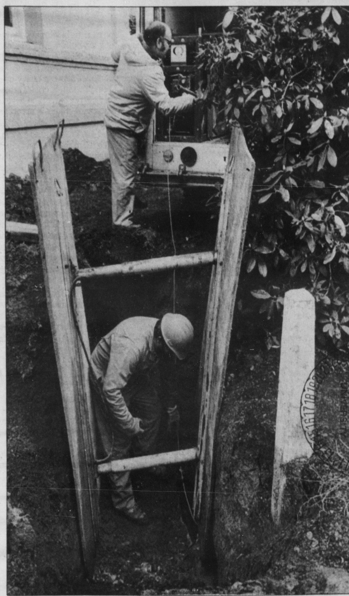
Workers of the Corvallis General Maintenance crew conducted an inspection of a sewer line outside Benton Hall Wednesday afternoon. The tile sewer line constructed in the early 1900's will have to be replaced.
