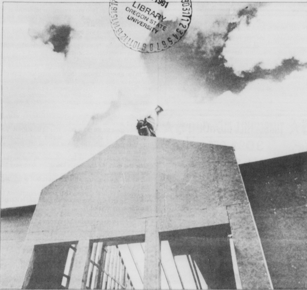
Norm Domagala of Dale Ramsay Construction enjoys a moment of sunshine while working on the rooftop of the new child care center behind Wilson Hall Thursday.
