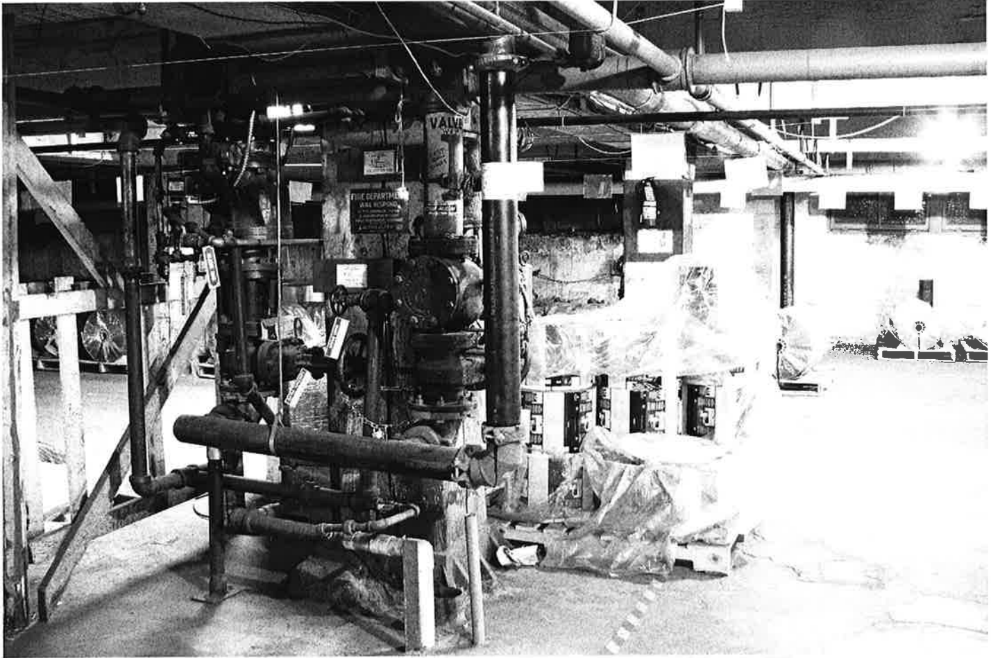
Photo 22 of 23: Basement: sprinkler equipment. View to SE.
