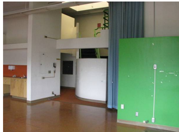
Main Building (370A), modern insertion of interior stair and room divisions on 4 th floor.
