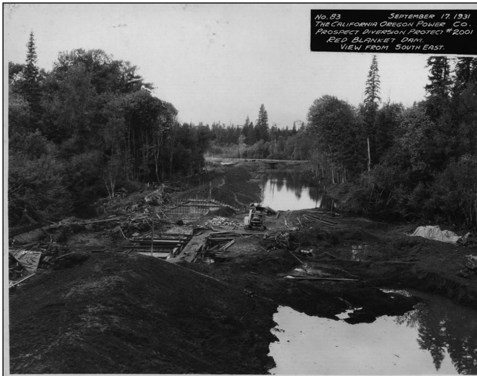
Figure 22. COPCO Prospect Diversion Project No. 2001, Photo No. 83, Red Blanket Dam, view from southeast, September 17, 1931.
