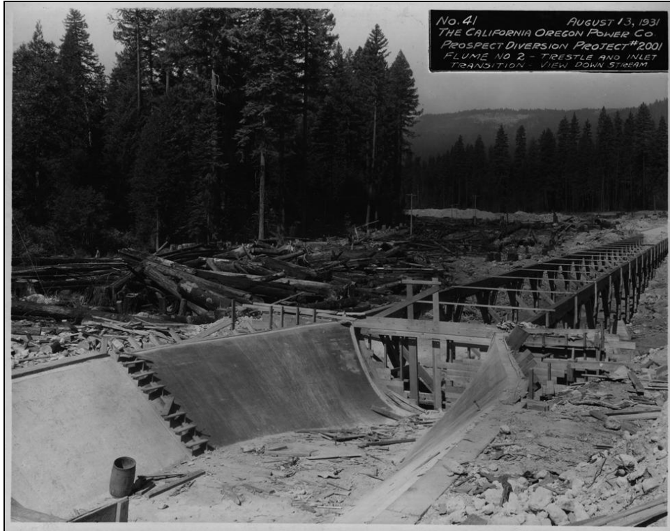
Figure 15. COPCO Prospect Diversion Project No. 2001, Photo No. 41, Flume No. 2 – Trestle and Inlet Transition, view downstream, August 13, 1931.
