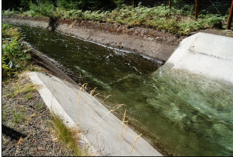
Figure 7. Typical view of the trapezoidal-shaped canal of the Prospect Diversion Project. Shown here, a relined segment adjoins the historic canal, 2009.
