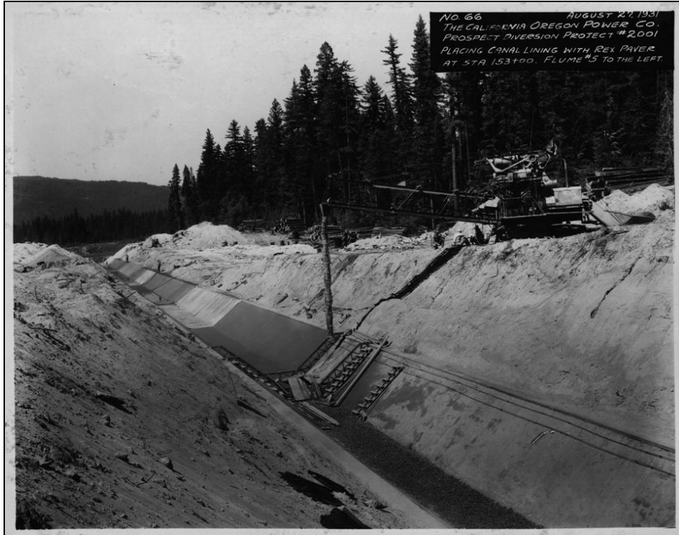
Figure 19. COPCO Prospect Diversion Project No. 2001, Photo No. 66, Placing Canal Lining with Rex Paver, August 27, 1931.
