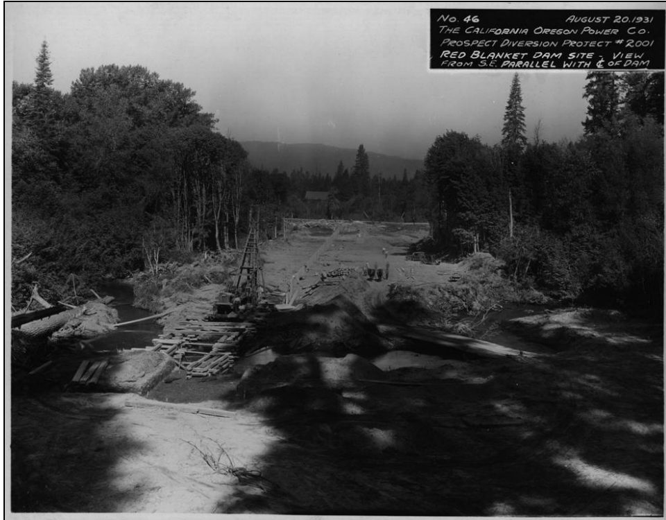
Figure 17. COPCO Prospect Diversion Project No. 2001, Photo No. 46, Red Blanket Dam Site – View from southeast parallel with centerline of dam, August 20, 1931.
