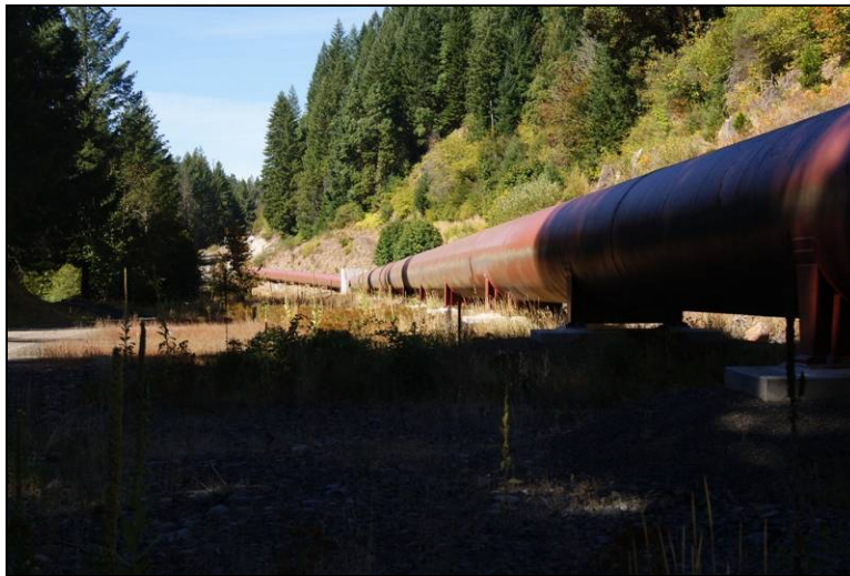
Figure 6. Enclosed steel pipe (also known as an inverted siphon) downstream of the Middle Fork dam, 2009.
