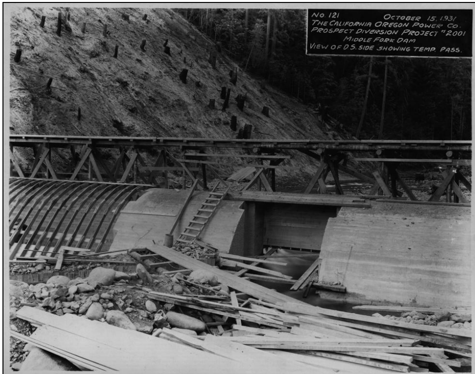
Figure 28. COPCO Prospect Diversion Project No. 2001, Photo No. 121, Middle Fork Dam, view of downstream side showing temporary passage, October 15, 1931.
