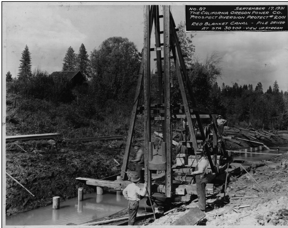
Figure 26. COPCO Prospect Diversion Project No. 2001, Photo No. 87, Red Blanket Canal Pile Driver, view upstream, September 17, 1931.
