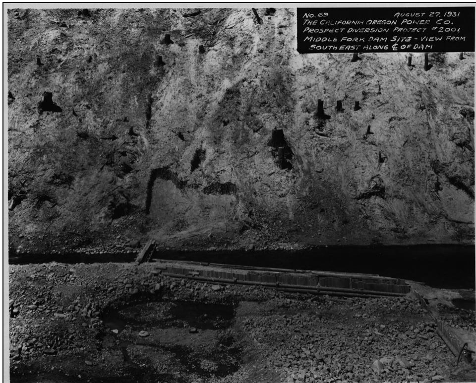
Figure 20. COPCO Prospect Diversion Project No. 2001, Photo No. 69, Middle Fork Dam site – View from southeast along centerline of dam, August 27, 1931.
