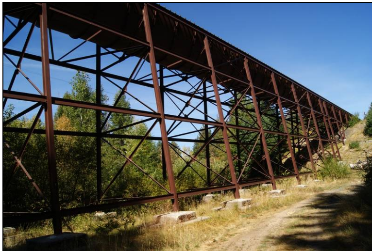
Figure 8. Steel flume, which replaced a wood flume of the same size, shape, and alignment. Note original concrete footings, which were reused for the steel flume, 2009.
