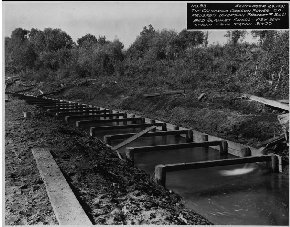
Figure 27. COPCO Prospect Diversion Project No. 2001, Photo No. 93, Red Blanket Canal – view downstream, September 24, 1931.
