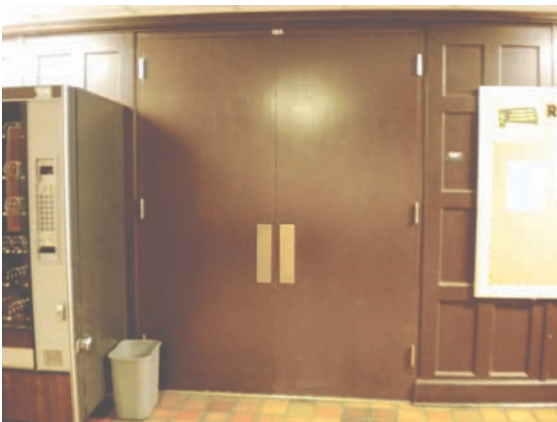
^ ROOM 154 - NEW (UNUSED) DOORS.
