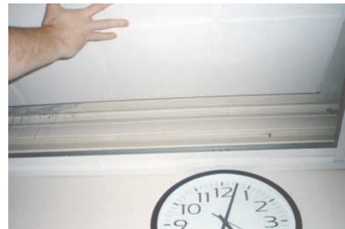
^ ORIGINAL WOOD TRIM ABOVE THE CEILING TILES.
