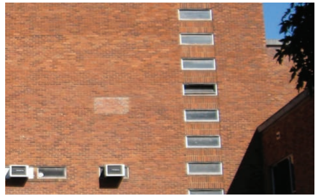
Infilled window on second floor at the time of 1985 addition of ballroom backstage.
