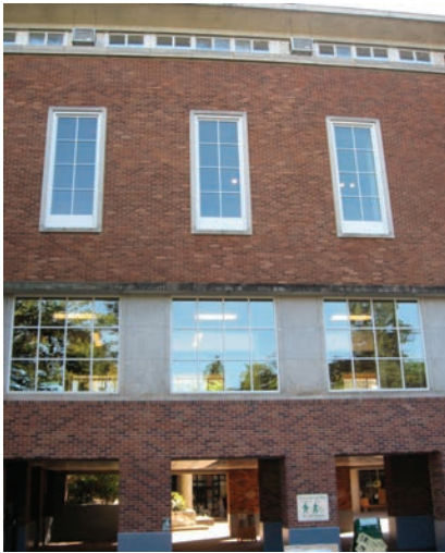
All existing openings and window frames & mullions are original. Breezeway excavation during 1973 addition.
