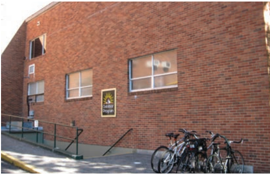
Ramp & rail extended, stairs to basement during 1962 addition. Windows original to this time.
