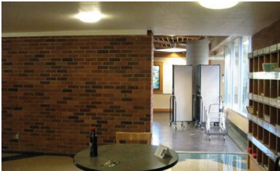
One of three openings in lobby cut in original exterior wall to make way for 1973 skybridge.
