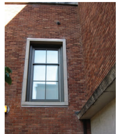
New opening for a window cut in south-facing wall to match existing during 2007 remodel.
