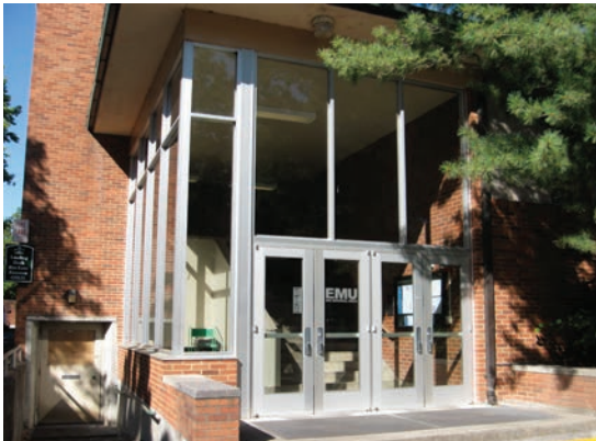
South Entrance aluminum storefront system replaced in kind in 2009. Original 1962 brick & limestone walls.
