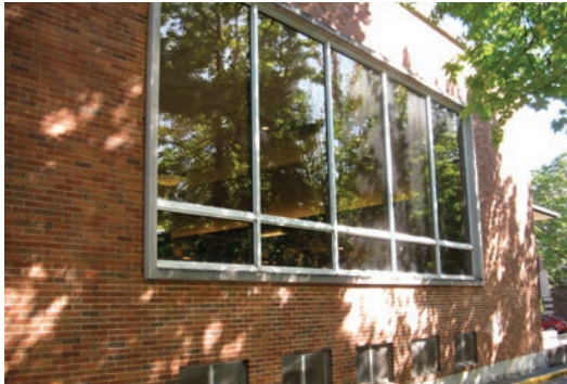
South Dining storefront windows replaced in 2009. Original vent openings below to basement.
