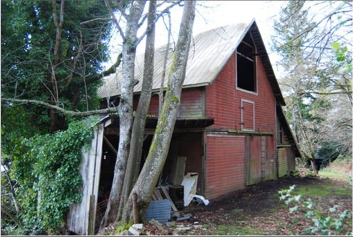
Photo 1 of 8: Looking northwest at the east façade with the south shed-roof addition in the foreground.
