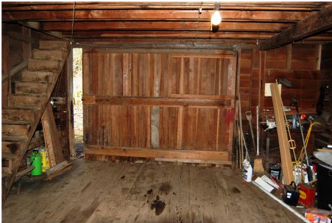
Photo 6 of 8: Looking east at the interior main mass, second floor, roller-door closed.
