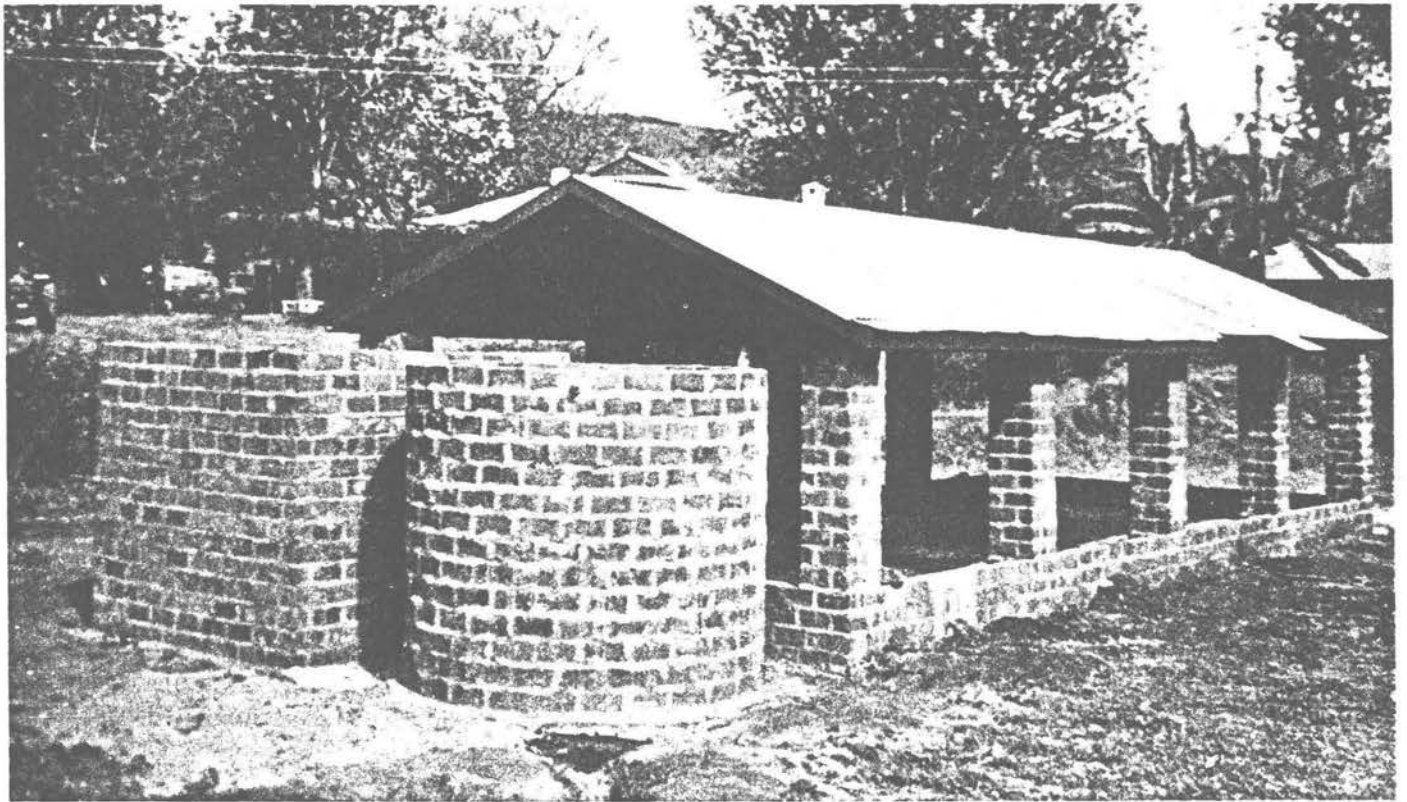
Specially developed brick tank reservoir to collect rainwater from tin-roof acting as micro-catchment area (see text)
