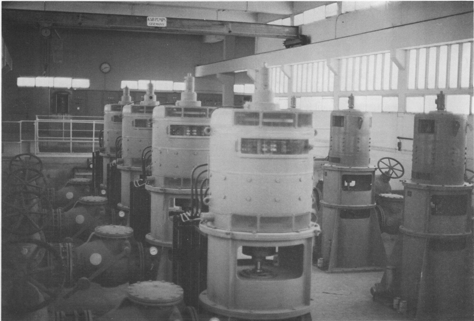
Figure 4 Electrically-driven vertical-spindle pumps, Benghazi Sewage Treatment Works, Libya.
