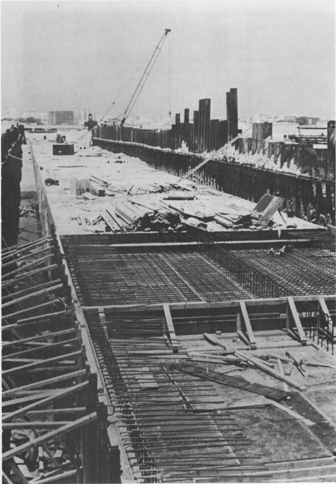
Figure 5 Twin 4 m x 2½ m reinforced concrete stormwater culvert under construction in Benghazi, Libya.
