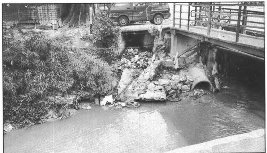
Low flows during droughts can also cause problems as the water velocities will be too slow to transport the wastes.
