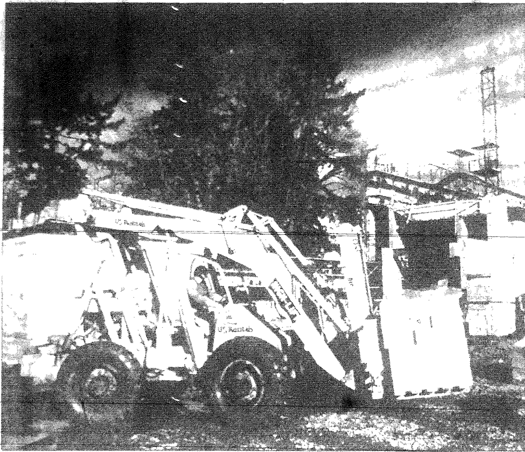
Construction continues on the new OSU Cultural and Conference Center located on the corner of 28th and Western. The center will be completed by next fall. Addition of this facility will help relieve scheduling conflicts and provide superior acoustics for musical and speaking events. (Photo by Fred Nelson.)
