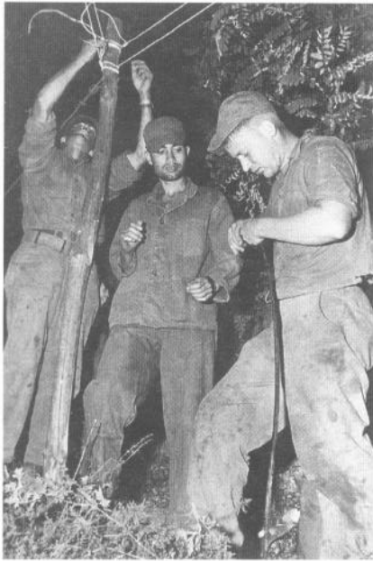
Navy Seabees (left to right) Electrician's Mates Troy Edwards, Julian Perez and Joseph D. Edson install floodlights on Red Beach at night on the 15th so that naval forces can sustain their critical over-the-shore logistics operations.
