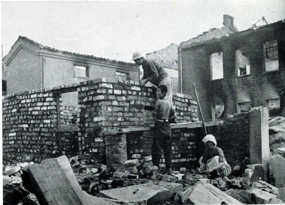
UNSKILLED HANDS WENT TO WORK AS KOREANS BEGAN THE BACK-BREAKING TASK OF RECONSTRUCTION
