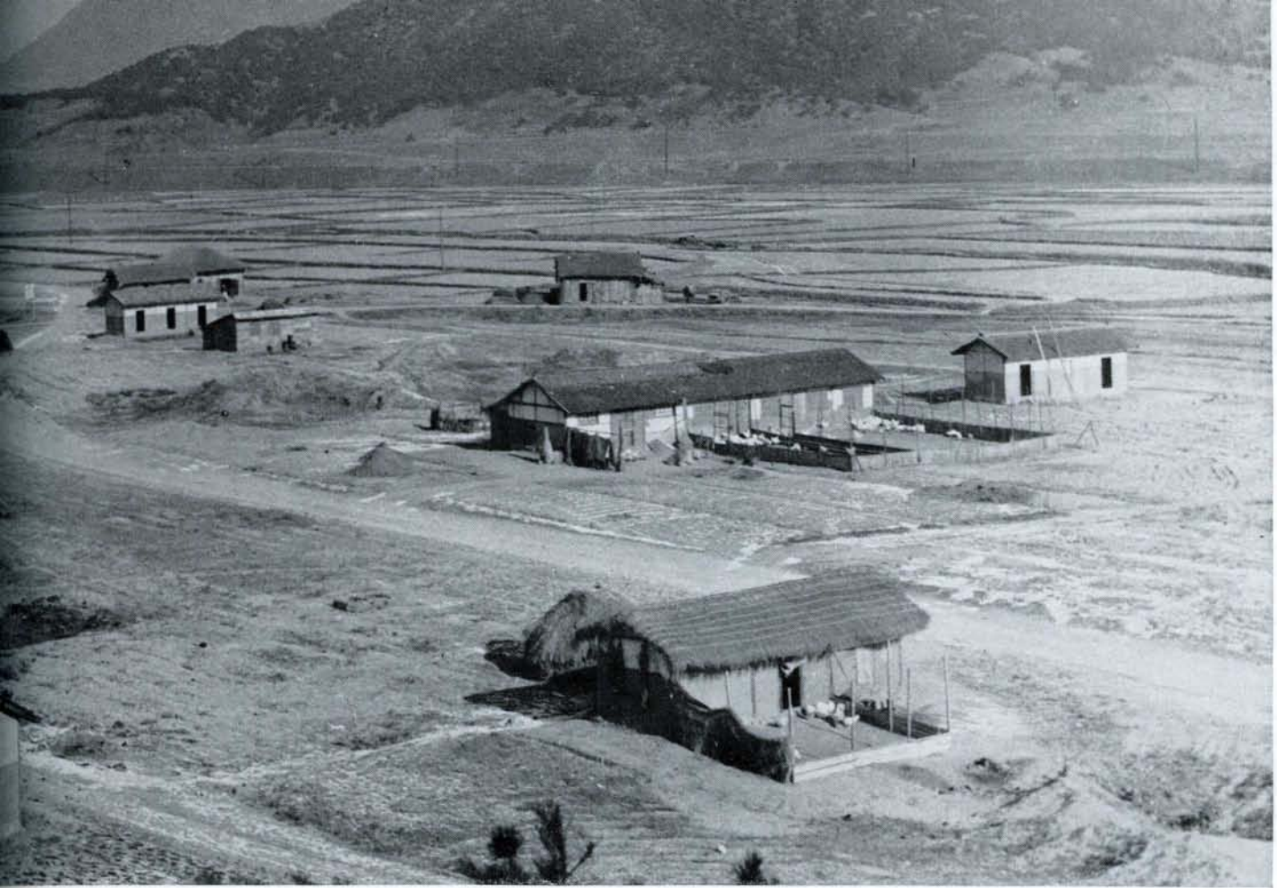
HOUSING PROBLEM. THE U. S. FURNISHED THE CONSTRUCTION MATERIALS FOR THIS REFUGEE HOUSING PROJECT BEING BUILT AT SHIN CHON.
