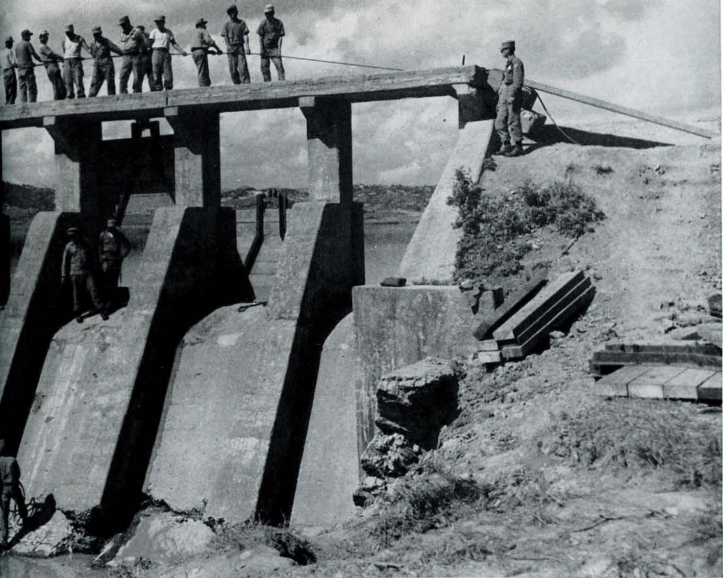
VOLUNTEERS IS ONE OF MANY U. S.-AIDED RECONSTRUCTION PROJECTS THAT WILL PROVIDE WATER TO IRRIGATE THE REPUBLIC'S RICE-GROWING VALLEYS.
