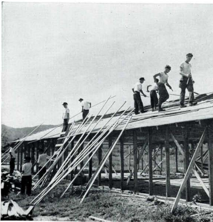
SCHOOL CONSTRUCTION UNDERWAY in 1952 with lumber purchased by UNKRA. Funds were appropriated by the United States Congress.
