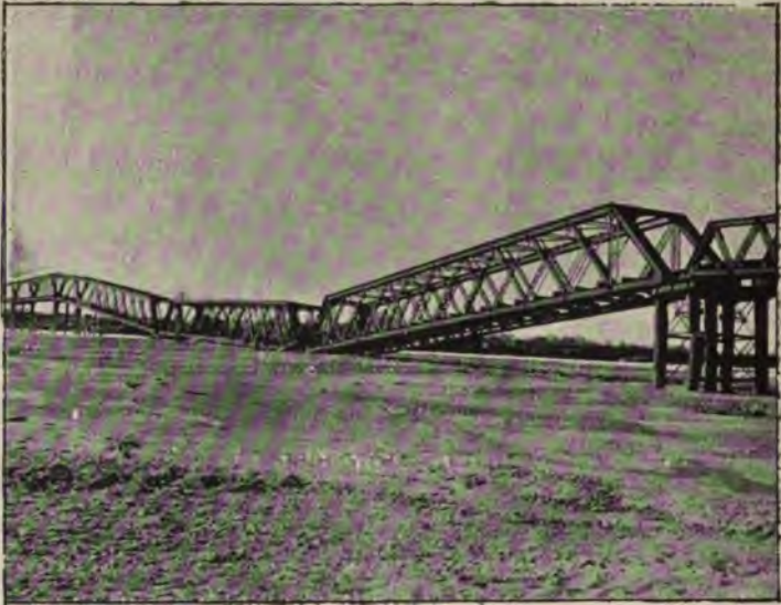
NAGARAWA BRIDGE AFTER THE EARTHQUAKE.
