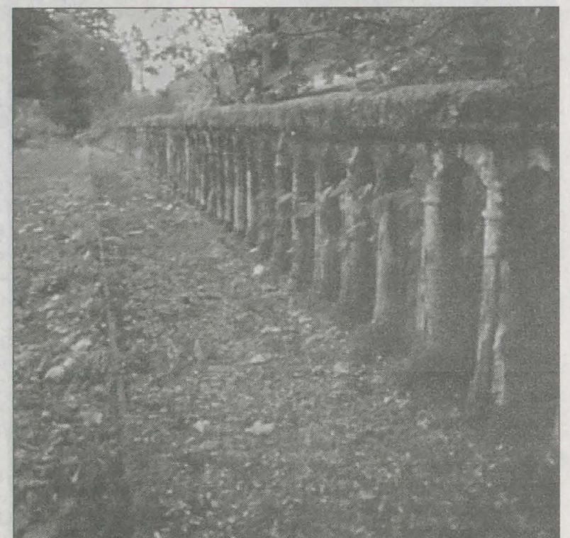
The abandoned Moffett Creek Bridge near Bonneville Dam. When constructed, it was the longest (170 feet) three-hinged, flat arch concrete bridge in the United States.
