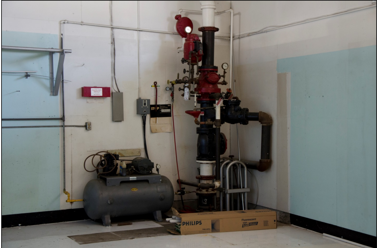
Photo 14 OR_MultnomahCounty_PortofPortlandHangar8005_0014 Fire suppression system in the west corner of Hangar 8005, view to the southwest.
