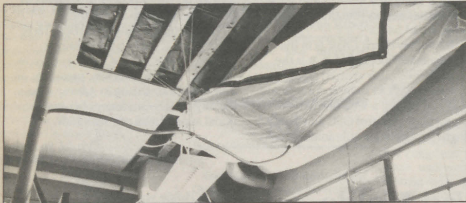
A "temporary" tarp installed to catch the drips in Wiegand Hall
