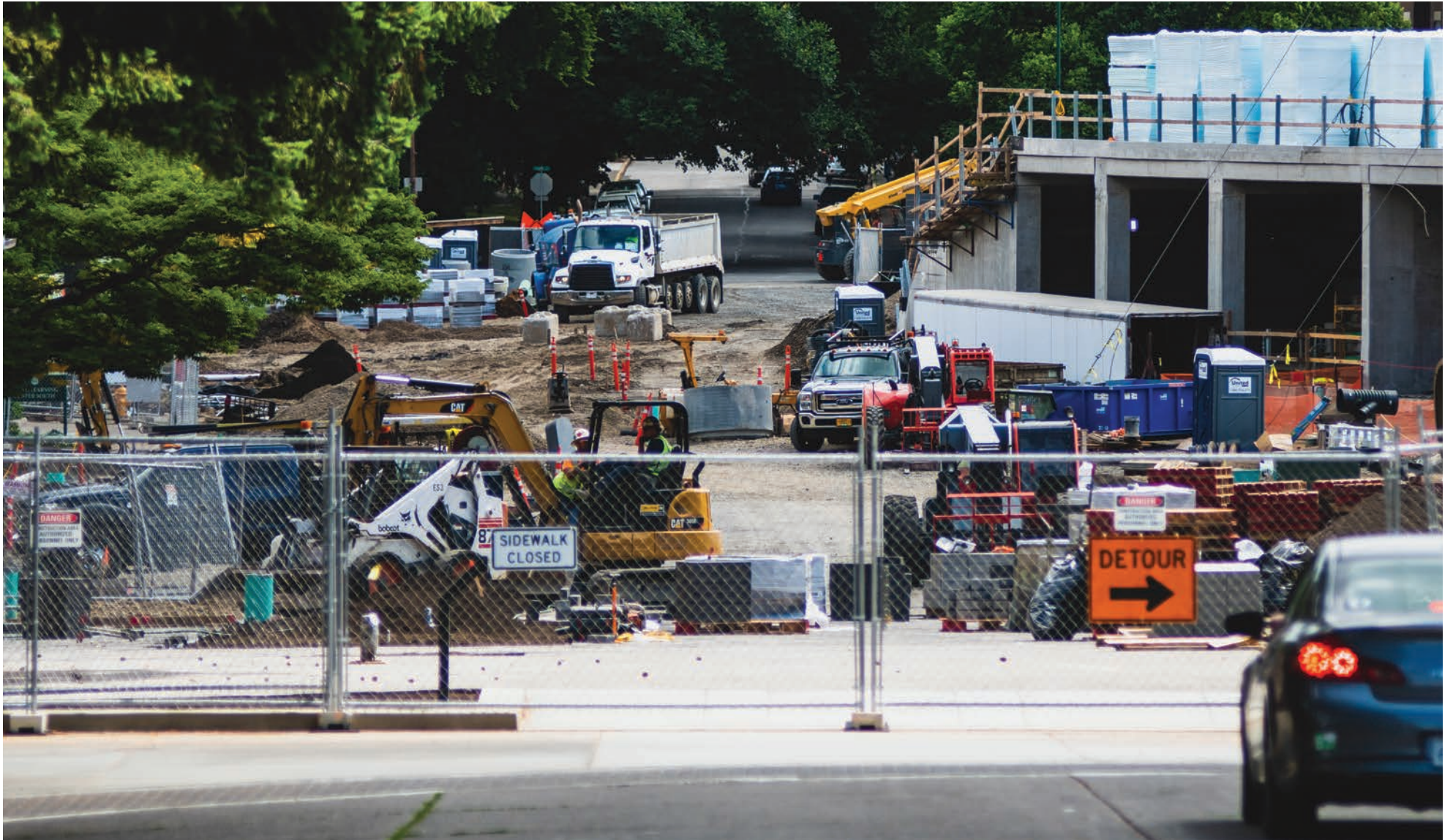
The construction of the new Hayward Field on the University of Oregon campus is limiting traffic along 15th. (Brad Smith/Emerald)
