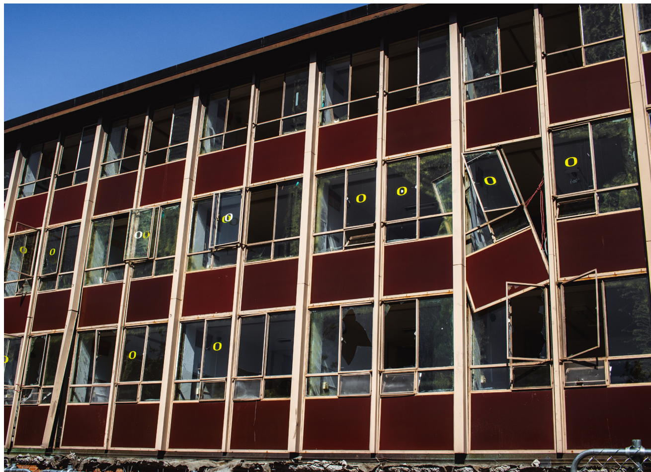
Walton hall lays in disarray during its demolition. The University of Oregon's oldest and most affordable residence hall, Walton, is currently being demolished (Will Geschke/Emerald).
