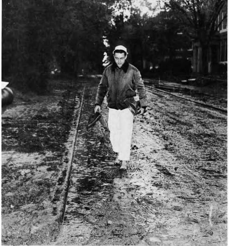
Zest for study is not squelched by mud-strewn streets of the campus. Getting to the library required ingenuity on student's part during installation of heating system.
