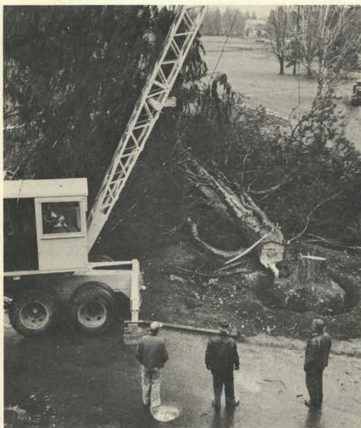
Construction crews remove a tree to prepare for the new street. The construction was first planned in the original campus layout.
