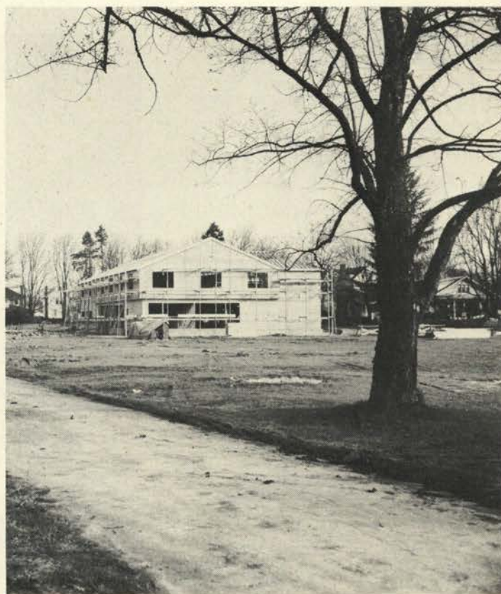
The new Azalea House, almost ready for the finishing touches, stands on lower campus. It will be ready for occupancy in the fall.
