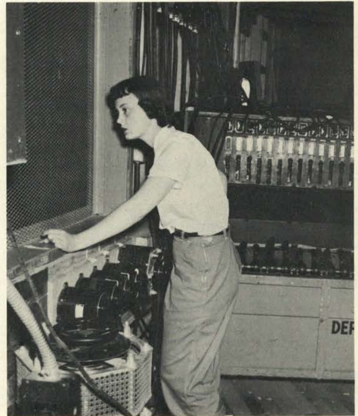
Controlling the lighting and effects for each play in the Playhouse is a student assistant. Production crew works with top quality equipment.
