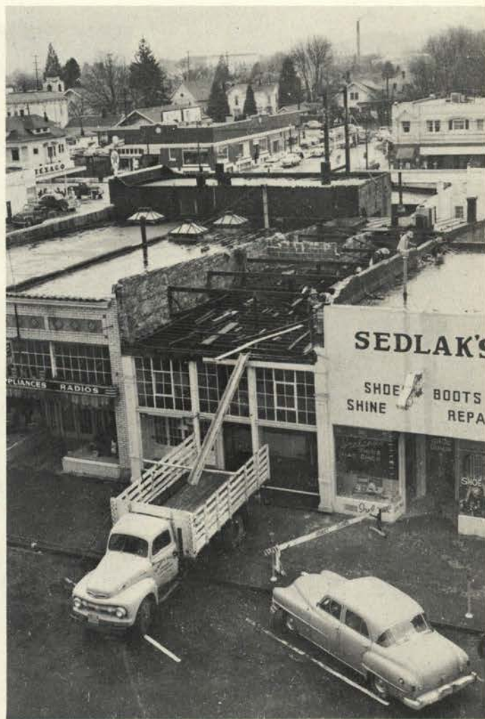
The false roof section of a shoe repair building toppled into the street and sidewalk below. The piece was about 10 feet high and weighed nearly a ton.
