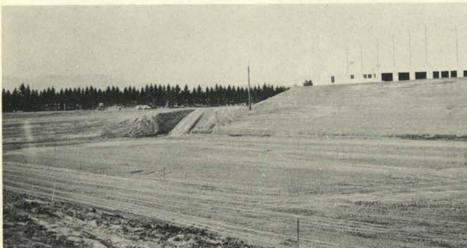
The stadium, completely excavated, waits for the field and concrete stands. It is built in the fashion of the Stanford Bowl.
