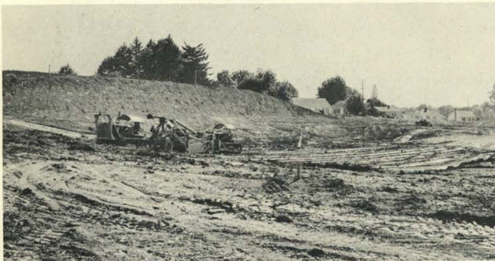
Giant machines excavate the new stadium site which will be finished this summer. The exceptionally dry fall enabled all primary work to be completed before the winter rains.
