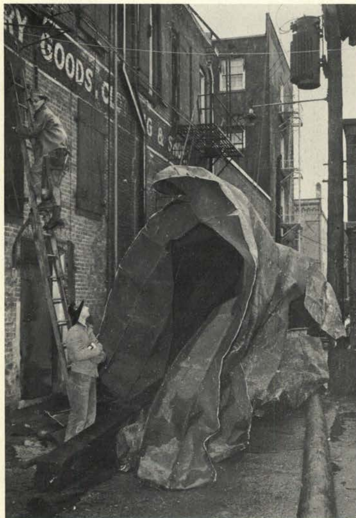
The roof of the Kline building in downtown Corvallis was blown off and landed in the alley behind, cutting power lines and knocking out transformers.
