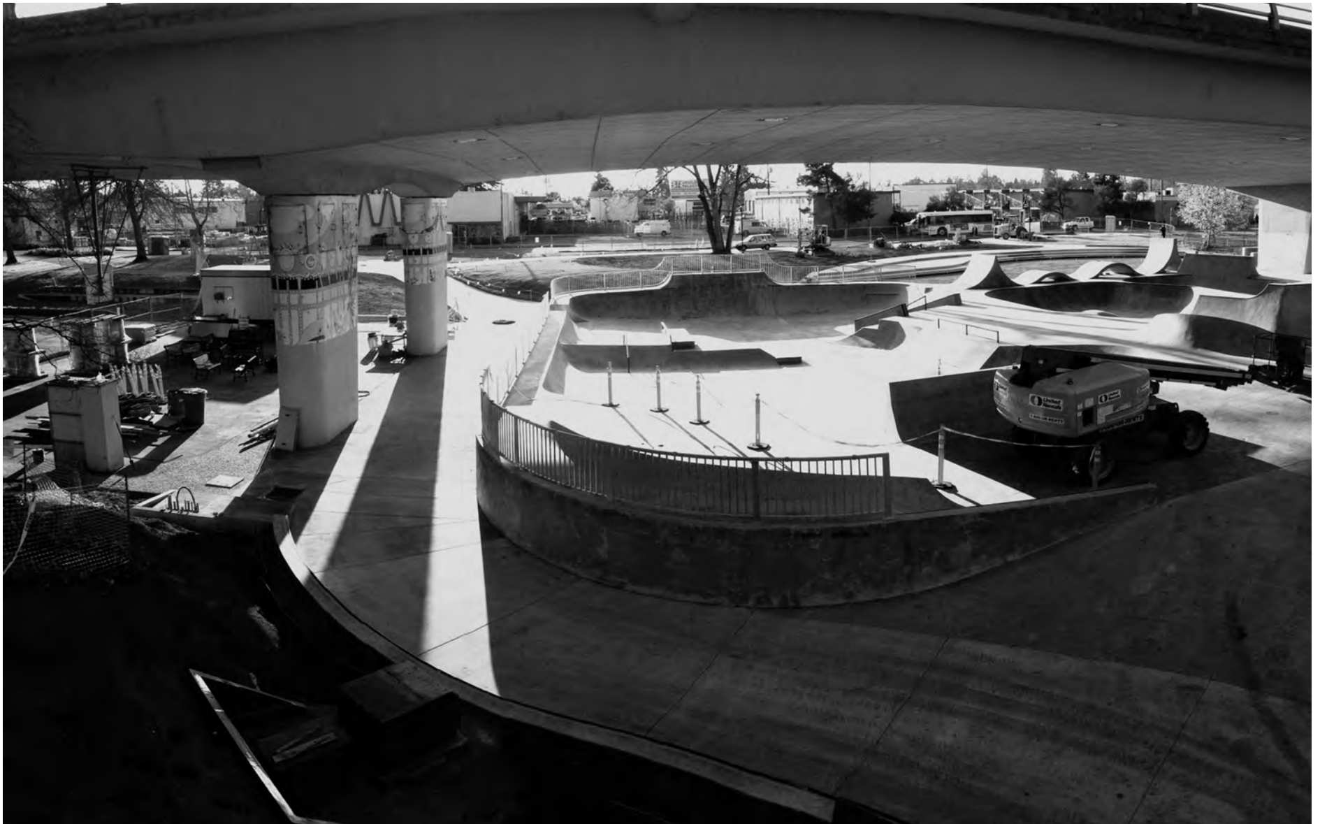
The Washington Jefferson Skatepark is under renovation to open in April with a grand opening in June.
