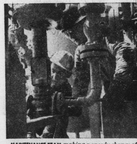
MAINTENANCE TEAM making a speedy change of a methanol valve to minimize production loss.
