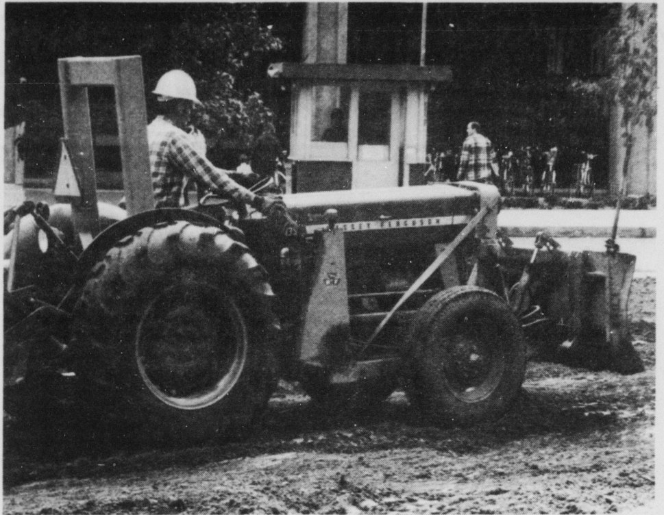
A bulldozer was busy clearing the area between the Administrative Services building and Ed Hall Friday afternoon. The area was occupied by two quonset huts recently torn down. The huts will be replaced by grass and shrubs soon. (Staff photo by Galen Momb)
