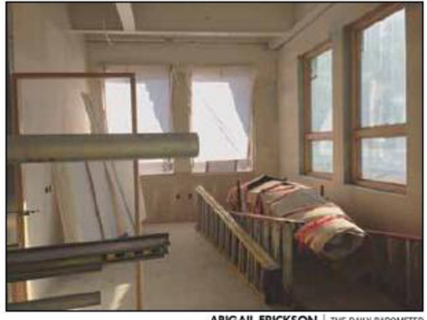
Light filters in through windows of an office on the fourth floor of the Student Experience Center.
