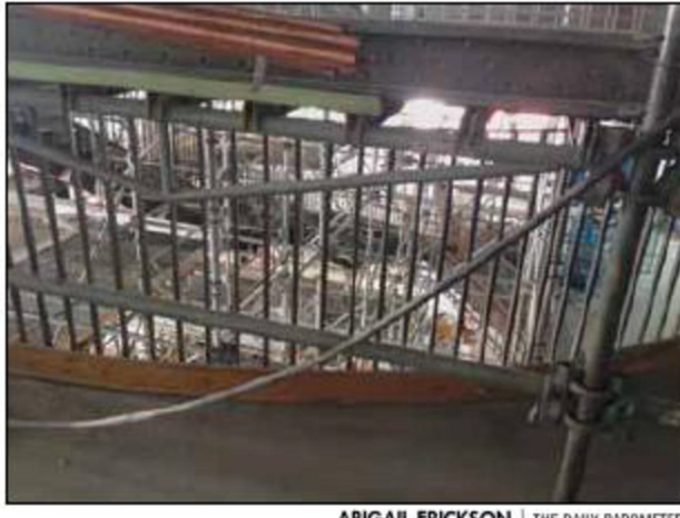
The center stairwell is visible while construction on the Student Experience Center continues.
