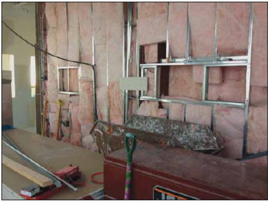
Metal frames mark the positions of television screens that will be placed in the fourth floor lobby of the Student Experience Center, the building under construction between the Memorial Union and the Oregon State University Valley Library. The fourth floor will be home to Student Media, including The Daily Barometer.
